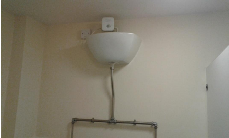
Flow Control to be replaced
