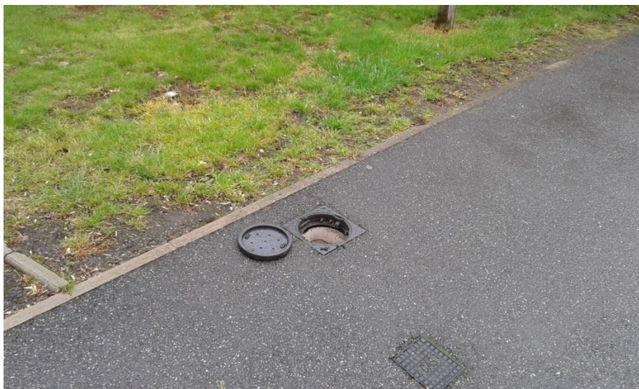
Meter in tarmac footpath by main gate
