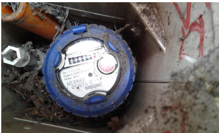
Meter in chamber
